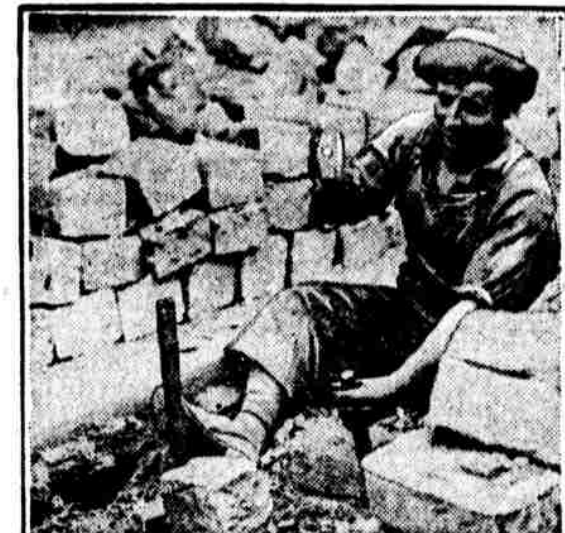
CUTS OLD BELGIAN BLOCKS IN HALF. Then they are dressed up a bit for use in the repaving of Sixth street
