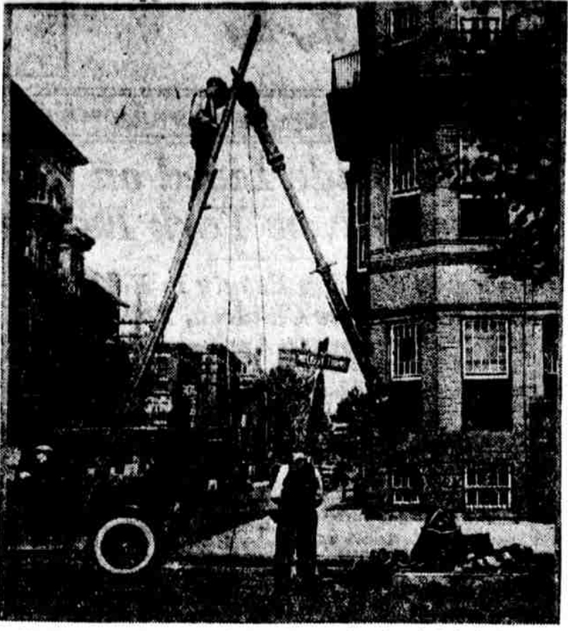
Workmen repairing an arc-light pole near Broad and Oxford streets after it had been hit by a heavy machine driven by Michael Berkowski, of Jersey City. Berkowski, arrested, says he lost control of the truck. He was not injured.
