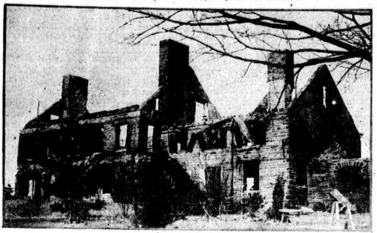
Only the walls remain standing of the home of Joseph Wharton Lippincott, at Bethayres, after a fire, which it is said the firemen were hampered in their fight by a lack of water.
