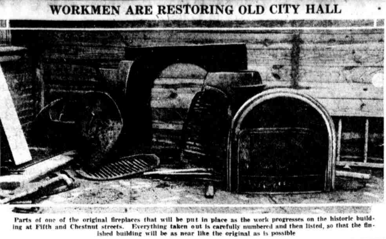
Parts of one of the original fireplaces that will be put in place as the work progresses on the historic building at Fifth and Chestnut streets. Everything taken out is carefully numbered and then listed, so that the finished building will be as near like the original as is possible.
