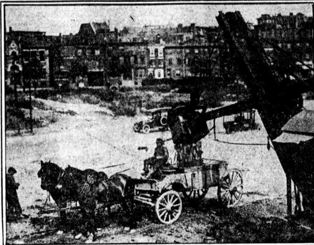
BUSY SECTION. A steam shovel scooping away the mountain of dirt at Twenty-fourth street and the Parkway. The dirt is being used for the Parkway foundation near the art gallery. Ledger Photo Service
