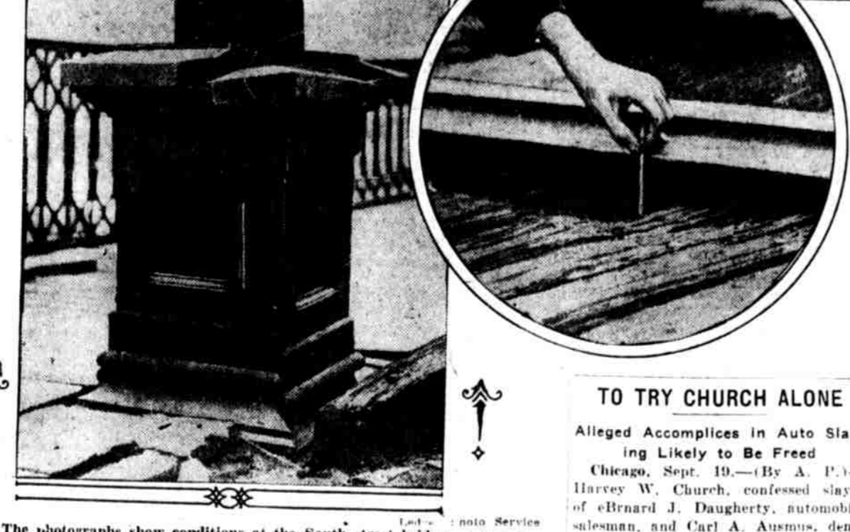
The photographs show conditions at the South street bridge—a sprung I beam, the trolley tracks sprung from the roadbed and loose, flapping girders.
