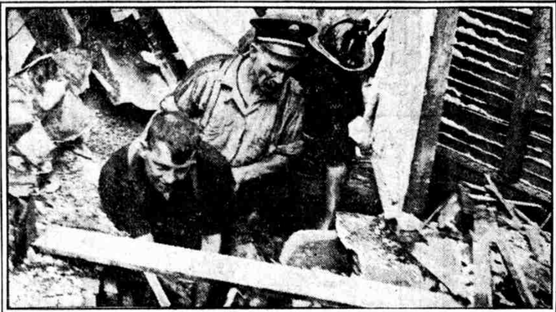
RESCUE WORK. Three city firemen removing debris as they make sure that no one is buried in the collapse of two houses at Sixtieth and Thompson streets, West Philadelphia. One man was rescued.
