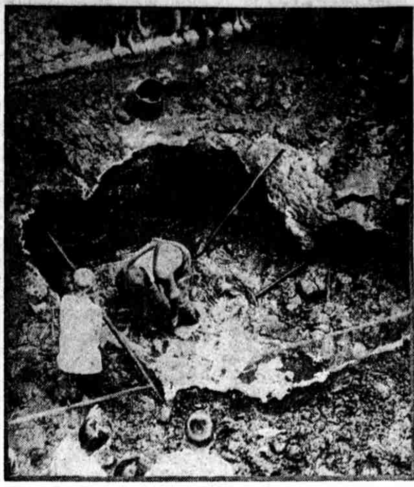
The picture shows how Salmon street caved in after a water main burst between Huntington street and Lehigh avenue. Water flooded basements of twenty houses, rising above the first floor in some. A workman is seen repairing the break.
