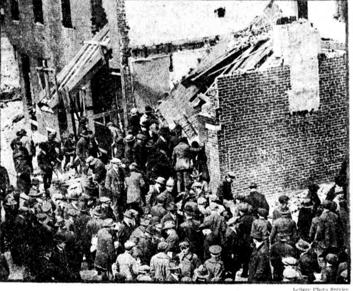
Scene at 2016 Winter street, where a sixty-year-old man met death, another employe was buried under debris, but dug out alive, and a foreman narrowly escaped death by clinging to a joist when a wall of a house that was being demolished collapsed about 11 o'clock this morning
