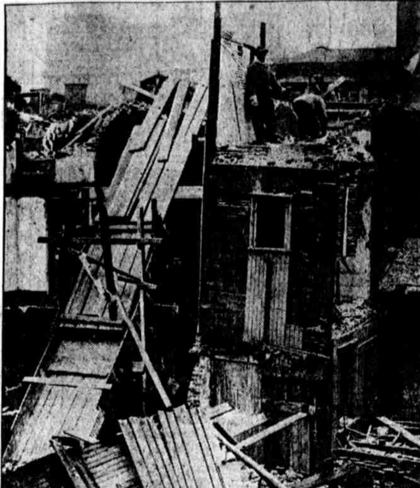
PASSING OF MANY OLD BUILDINGS. They are being taken away to make room for another recreation center, where the children in the neighborhood, of Eleventh and Rodman streets may play out in the open. Ledger Photo Service.
