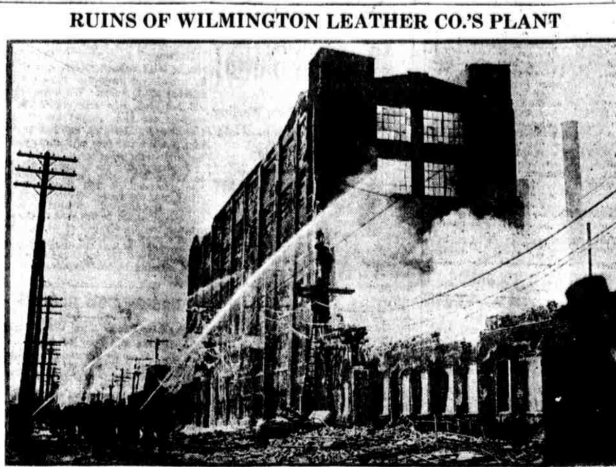
Blackened walls and great masses of warped and twisted iron pipes and girders are all that remained today of the big tannery owned by the Wilmington Leather Co., which was burned yesterday with a loss estimated at approximately $3,000,000. A large quantity of raw material and manufactured products was destroyed, together with six residences.
