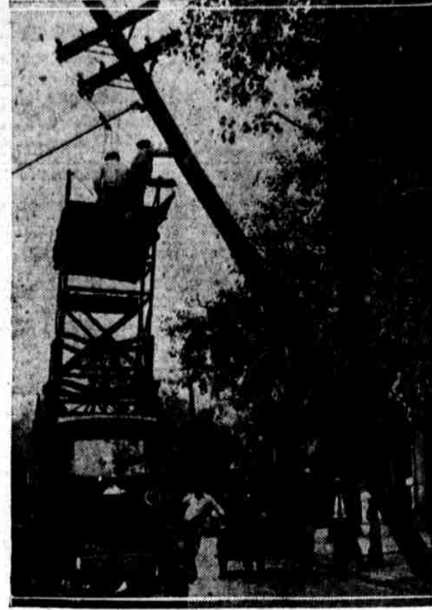
POLE BROKEN BY STORM FALLS TWELVE HOURS LATER. The pole at Thirty-sixth and Chestnut streets carried Philadelphia Electric Co. power lines, which are holding it up.
