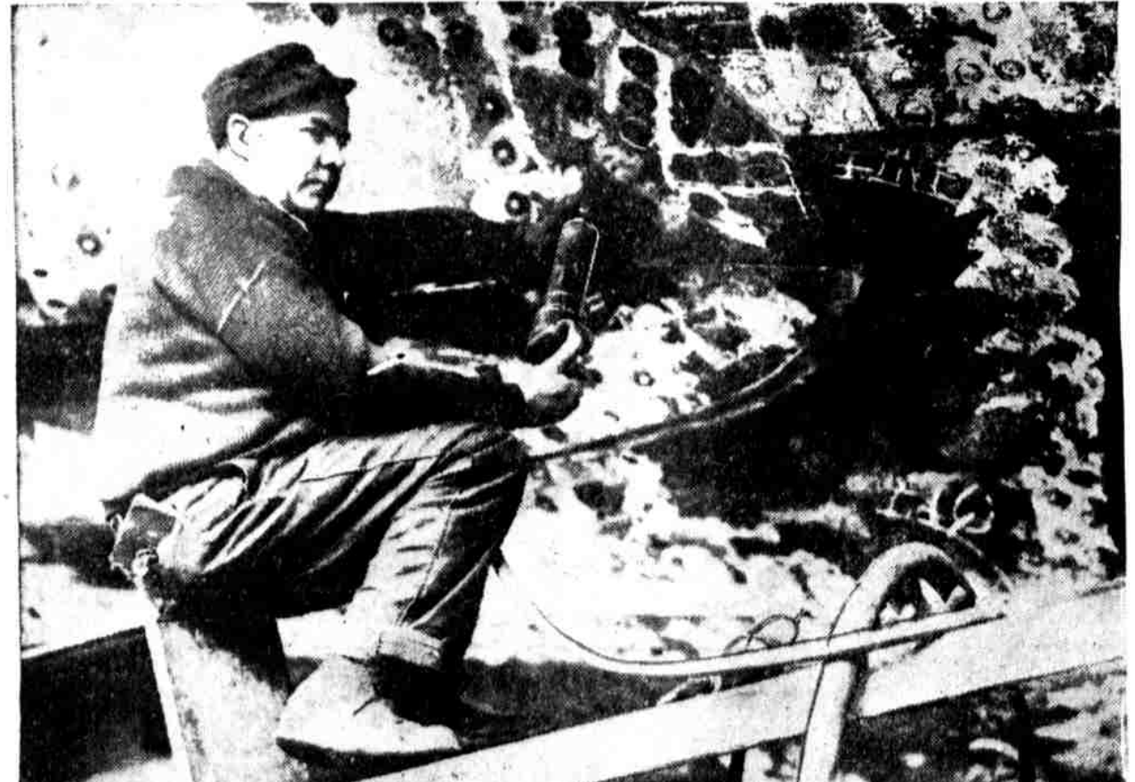
RIVETING BOILER PLATE. The workman is Christopher L. Paul, foreman of riveters at the New York Shipbuilding Co., Camden. He has been a riveter since the opening of the shipyard
