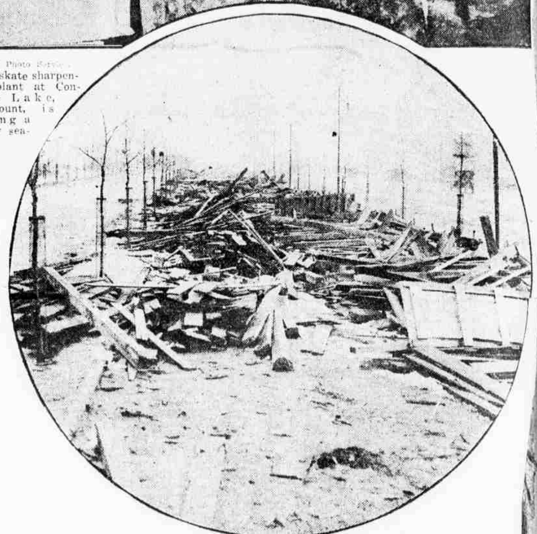
CITY workmen are busy tearing down the grandstands along the Parkway. They were used at the parades during city's war activities.
