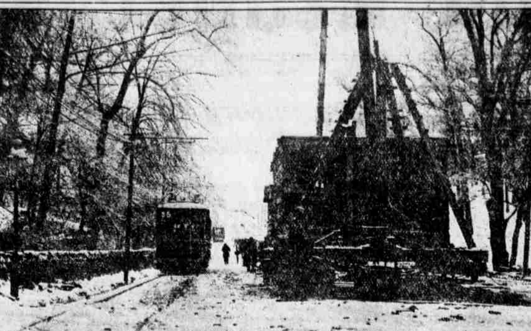
Illustrations show spot on York road just below Chelten avenue where the excavation for the construction of an extension of the Rock road sewer is located and which has been closed to traffic.
