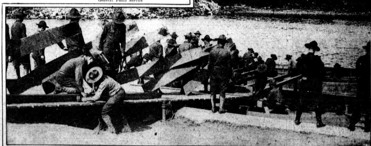
SOME DAY TO BRIDGE THE RHINE is the dream of the American engineers here experimenting in constructing a crossing over the Potomac. Note how many different tasks are being undertaken at one and the same time.
