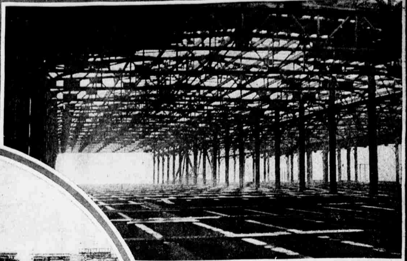
A View of Municipal Pier No. 78 at the Foot of McKean Street, Which, Although Not Yet Completed, Has Been Leased by the Government as an Outlet for the Two Great Overseas Supply Depots in Course of Construction Here.
