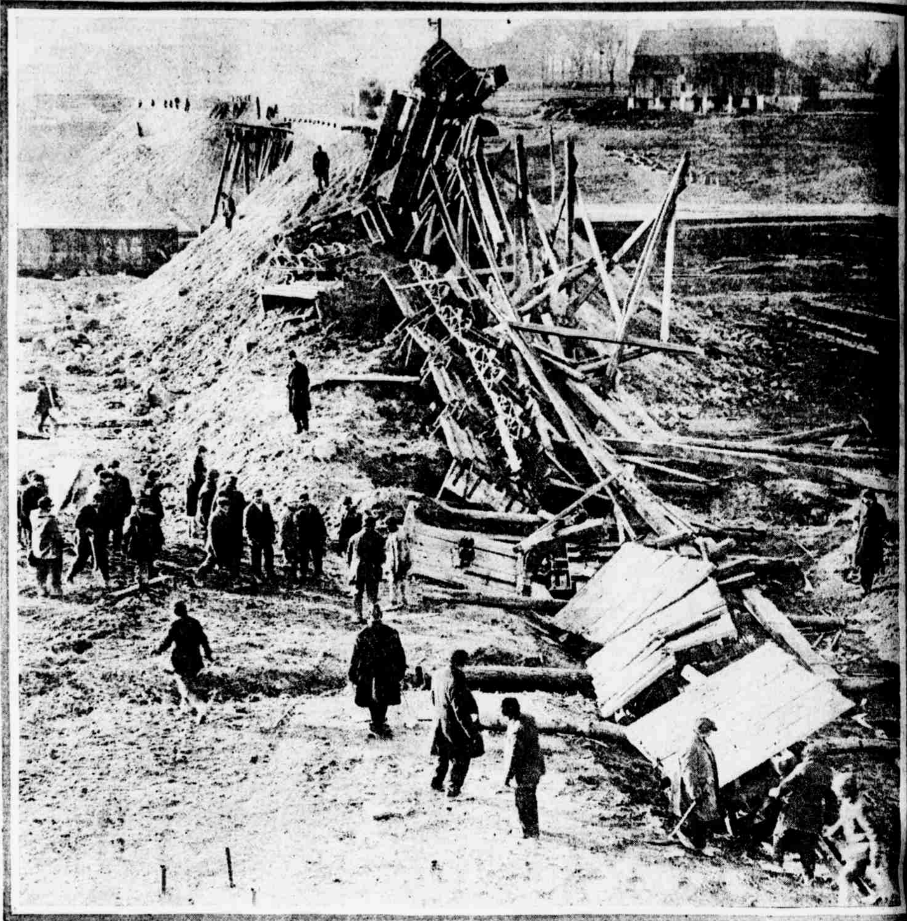
When a Trestle of the Small Bridge Being Constructed by the Pennsylvania Railroad at Sixtieth Street and Eastwick Avenue Gave Way Late Yesterday Afternoon Four Narrow-Gauge Cars Loaded With Building Material Rolled Into the Excavation and Buried Ten Workmen Beneath the Debris. Four of the Men Were Instantly Killed and Three Others Seriously Injured.
