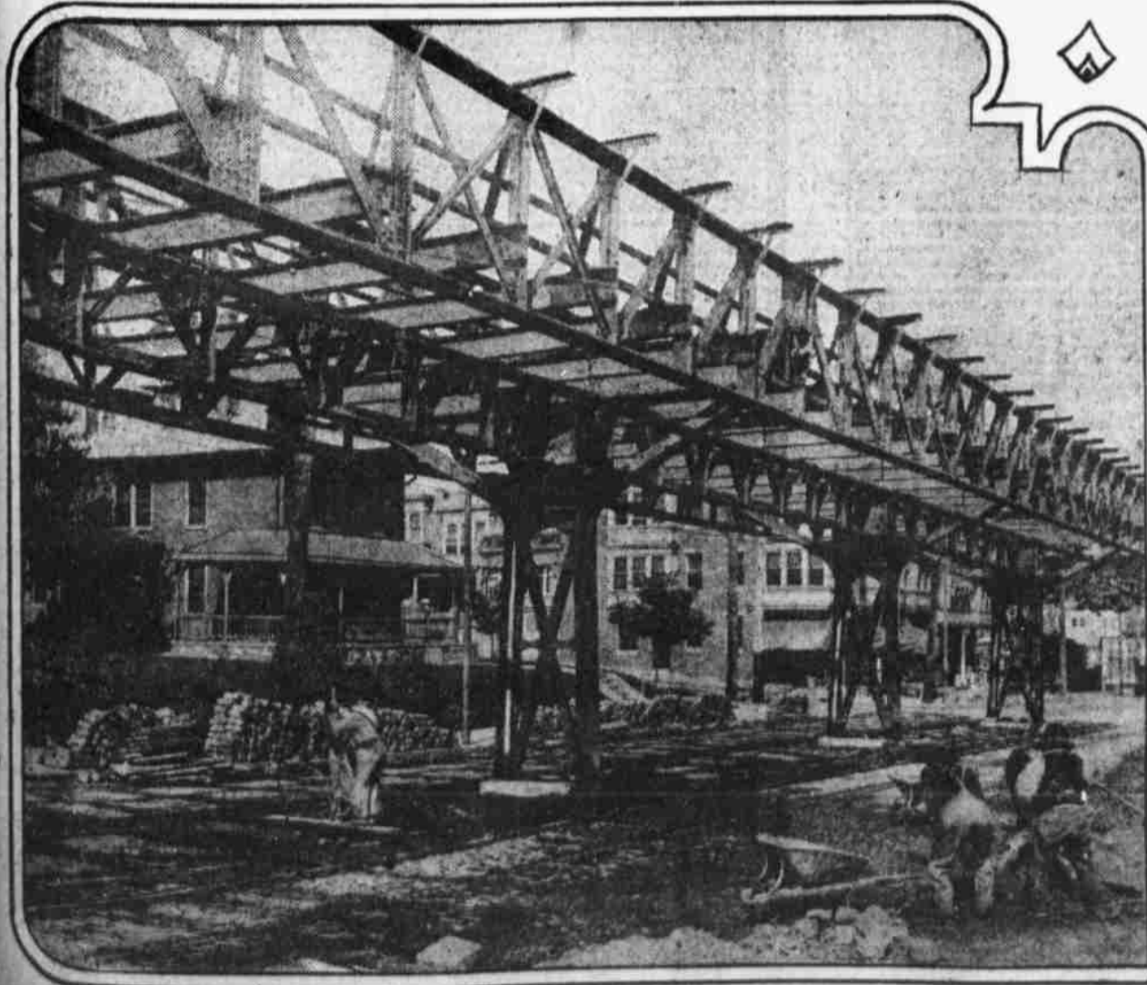
SUPERSTRUCTURE FOR NORTHEASTERN OVERHEAD LINE NOW EXTENDS TO DYRE STREET Though progress is not so rapid as ardent advocates may wish, there is tangible evidence of gradual accomplishment.
