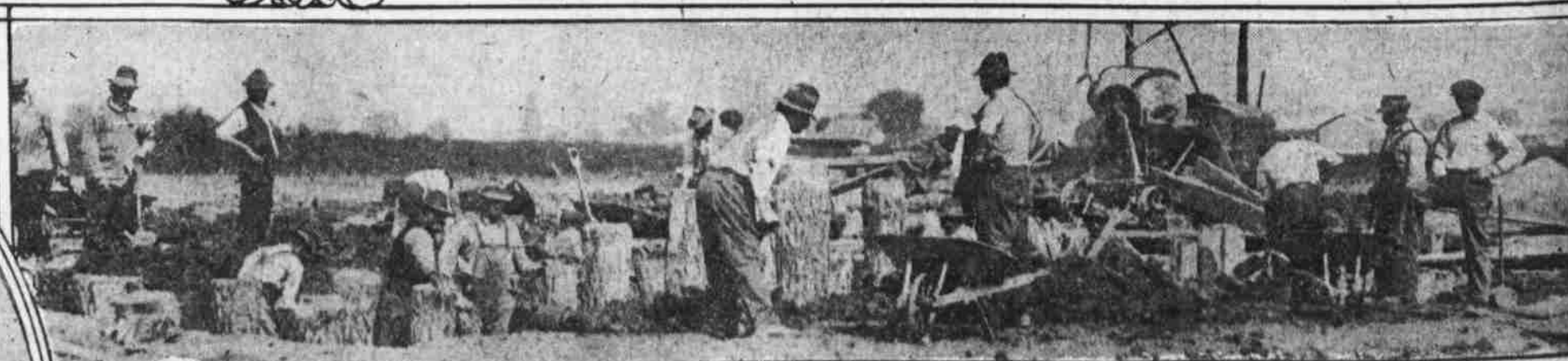
LAYING FOUNDATIONS FOR THE RAILROAD SPUR WHERE IT WILL CROSS THE ERSTWHILE BED OF A CREEK
