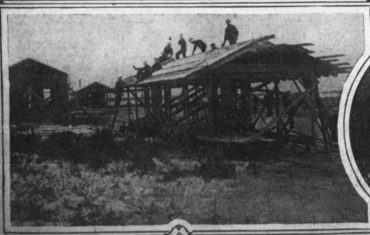
RESERVISTS BUILDING OBSERVATION HOUSES FOR THE RIFLE RANGE And making a good job of it, too. A few months ago these lads were book clerks, salaried men and the like. Before enlisting most of them were unused to manual labor.
