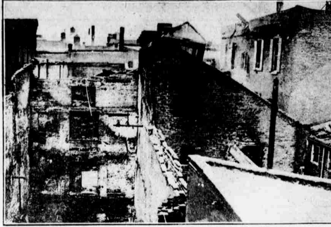
More than $50,000 damage was done early today by fire which virtually destroyed the building 114 North Front street, occupied by George D. Wetherill & Co., paint manufacturers. Only the walls of the structure remained and adjacent properties were damaged. An explosion preceded the fire.
