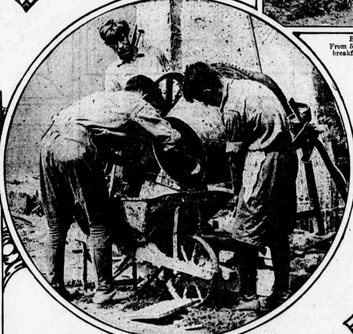
THE SCOUTS ARE EXPERT WORKERS IN CONCRETE The lads in the picture are mixing stones and cement for the floor of a large shower bath they are constructing. Already they have built a concrete floor for the barn they have turned into a habitation. Next they plan to construct a huge hen house with concrete steps and floors.
