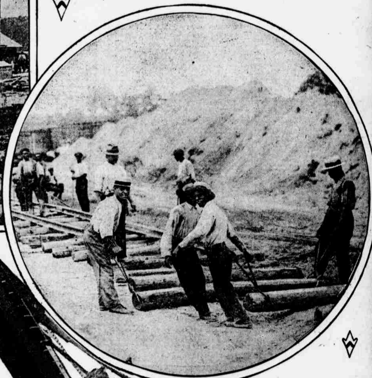
Scores of laborers are engaged in building sidings and spurs that will bring the encampment into direct connection with the Baltimore and Ohio system at Annapolis Junction.
