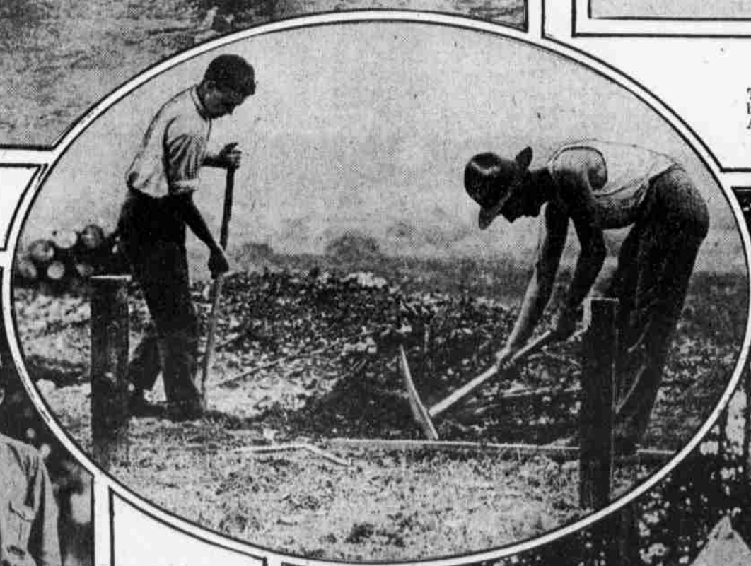
Cadets of the Hill School at Pottstown laying a drain on the outskirts of their encampment.
