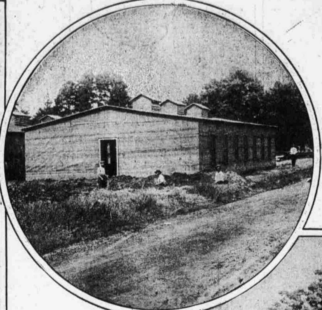
Eight of these workmen's bunkhouses are nearing completion, and work on more of them is going forward at top speed.
