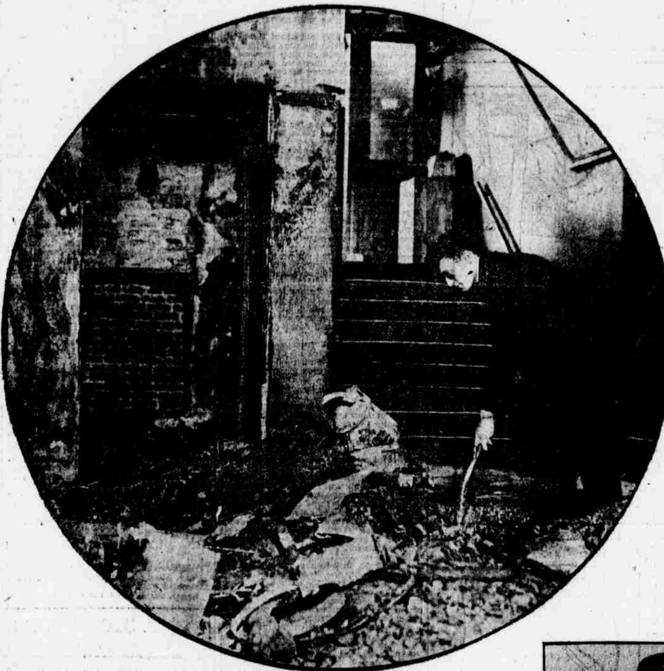
GAS EXPLOSION WRECKS WEST PHILADELPHIA SCHOOL Serious damage was done early today to the William B. Hanna building, at Fifty-eighth and Media streets, the interior of the structure being badly shattered in places, forcing temporary suspension of sessions to the delight of several hundred pupils.
