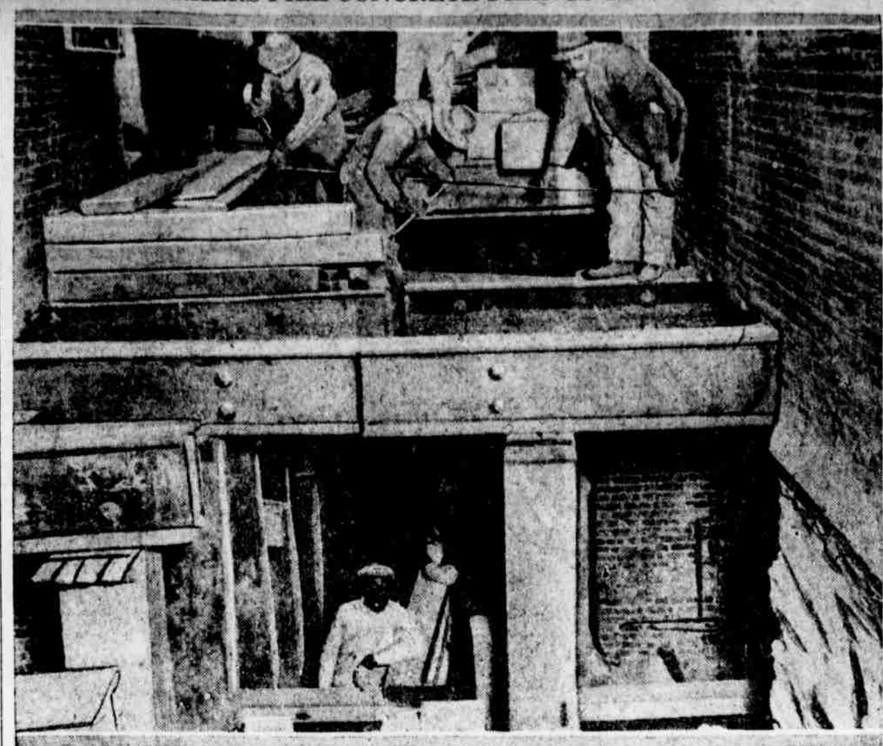
On the right, the vertical wall is part of the foundation of City Hall under the south corridor. In order to reinforce this against the shock and vibration caused by passing trains, wooden troughs are sunk at intervals into which concrete is placed and allowed to harden.
