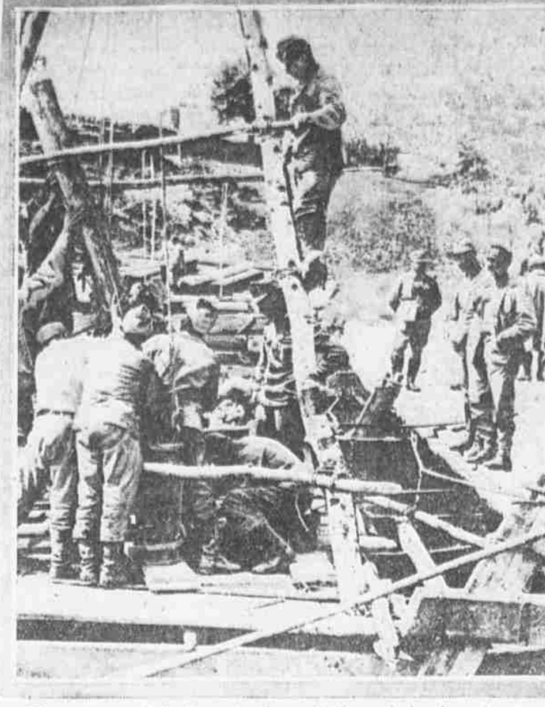
The swiftness of the Teutonic advance in Rumania has been due in no small part to the efficiency of the Austro-German engineers, who are equipped to meet all emergencies. The picture shows a skeleton bridge being thrown across a stream.
