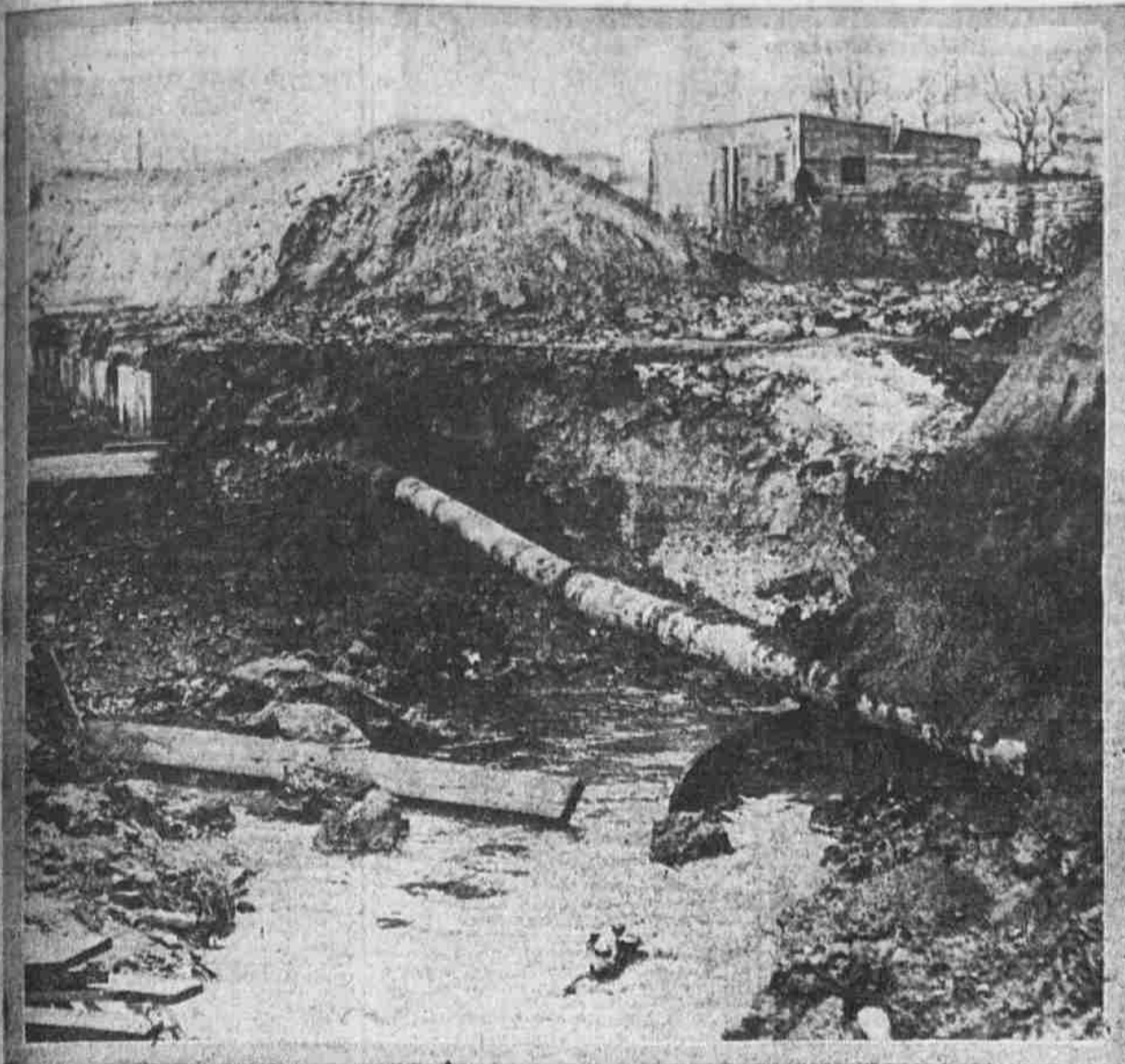
All of Philadelphia east of Broad street and south of Kensington avenue and Frankford Creek found itself without water today because of a broken 48-inch main at Wheatsheaf lane and Jasper street. Excavations for a sewer, it is believed, so weakened the support of the main that the pressure of the water caused the huge pipe to burst. The first rush of water broke down the boarding on either side of the sewer excavation and undermined the surrounding mounds of dirt and rock. The main split lengthwise, like an egg shell. A portion of the main is seen at the right of the picture.
