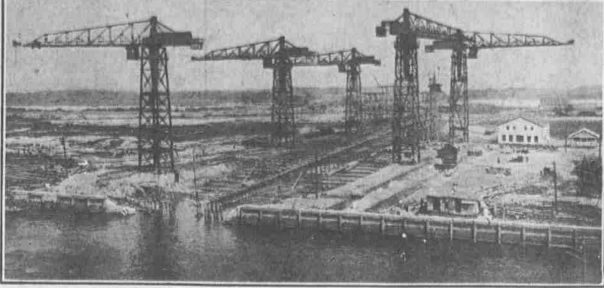
The completion of these ways, started on September 22, 1914, means the transformation of the navy yard from a repair station to a shipbuilding yard. Here a new building will build army transport No. 1 at a cost of $1,500,000.
