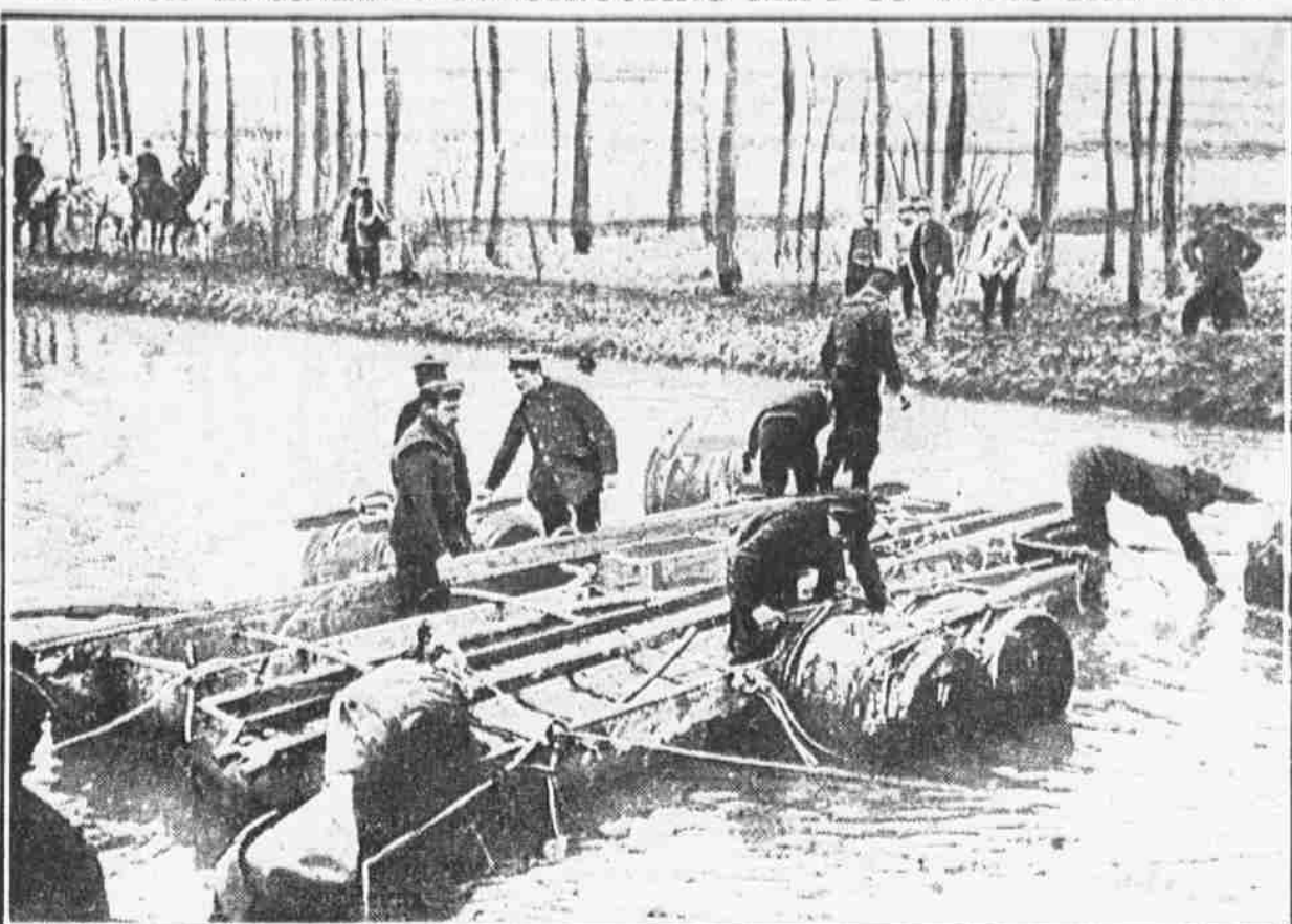
A squad of French engineers is seen building a temporary bridge across the Yser. In this region some of the bloodiest fighting of the war has gone on, as the desperate charges of the Allied forces have been met with energetic resistance by the Germans.
