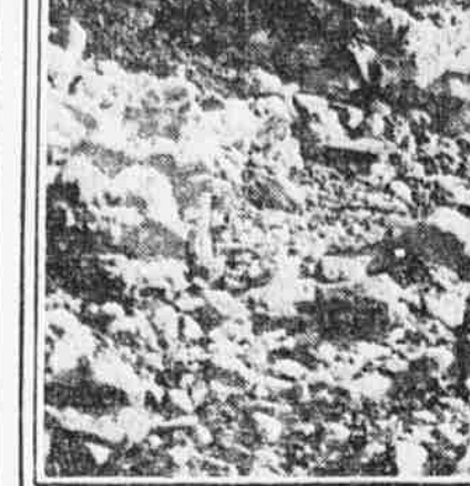
PART OF "NEAR CONCRETE" WALL DEFENDED BY EDWIN H. VARE. WALL IS NOW BEING TORN DOWN
