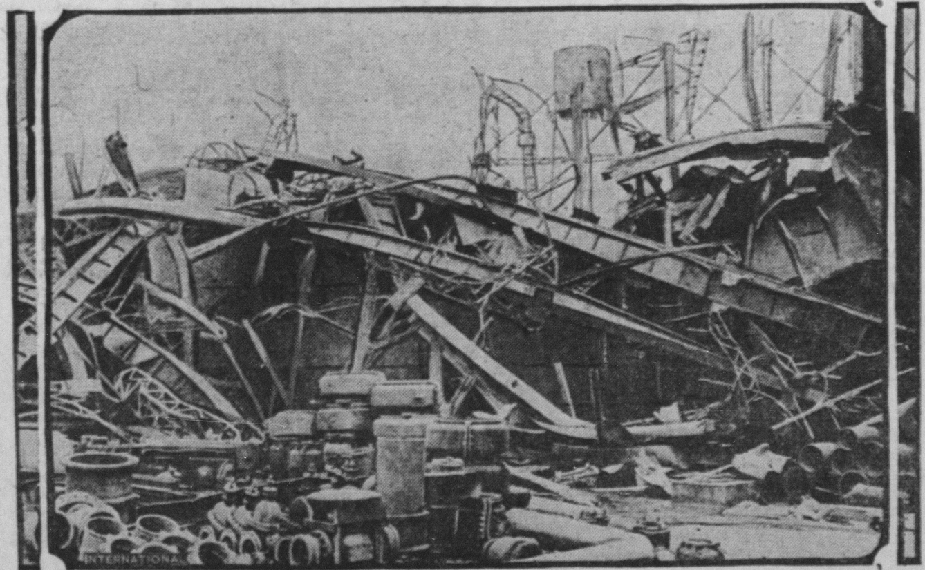
One of the big buildings that was wrecked by the terrific gas tank explosion in Pittsburgh, Pa. Scores of lives were lost and hundreds of persons were injured, while the property losses were immense.
