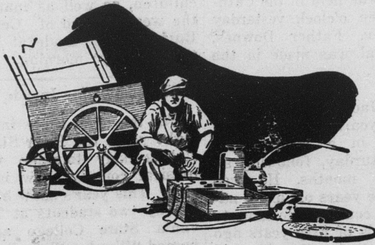
More than 2,000,000 miles of underground wires must be carefully and constantly tested to insure an uninterrupted service
