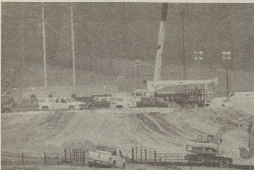
Natural gas drilling is booming all over the Commonwealth, and drilling sites, like this one in rural Bradford County, have come under scrutiny regarding safety. Penn State is partnering with other universities across the country to develop a training program for people working in the fast-growing natural gas and oil development industry. (photo credit C.J. Marshall)
