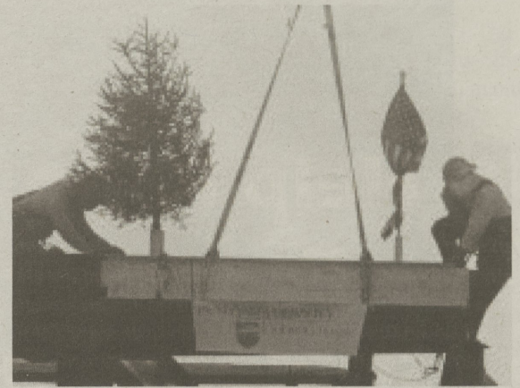
Construction workers place the final beam on Penn State Hershey Children's Hospital. This occasion marks another major step toward completion of the facility, slated to open in late 2012. (photo courtesy of Penn State University)
