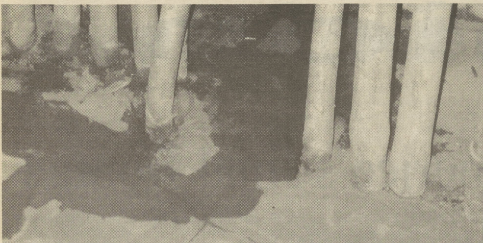
Basement floor of Classroom building, pipes containing electrical wires surrounded by water.
