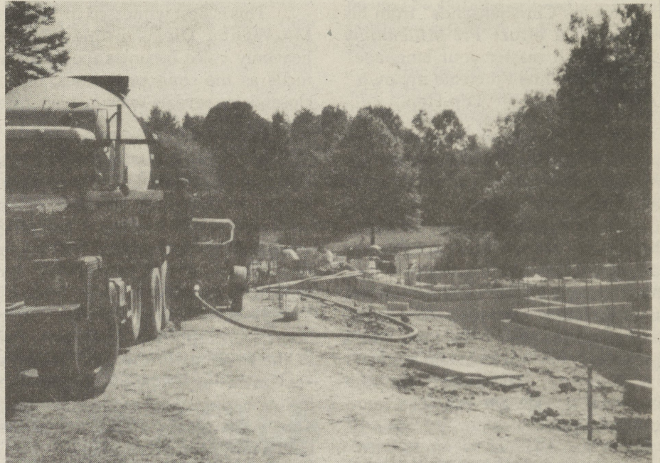
Construction of the new technology center continues, funded in part by Operation Jump Start, Bell Atlantic PA and Boeing Helicopters.
